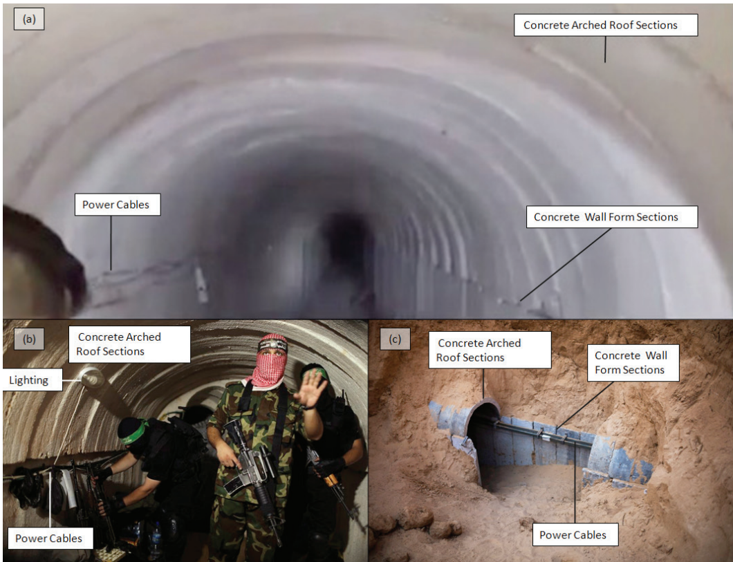
Figure 2. (a). Tunnel in Raqqa captured on the 5th September, 2017 from Da'esh constructed with prefabricated reinforced concrete 115 . (b). Tunnel in Gaza captured in August 2014 116 with characteristics similar to that shown in (a) captured in Raqqa . (c). Tunnel in Gaza captured by IDF Nov 2014 117 showing how concrete forms are used in tunnel lining similar to that shown in (a).
